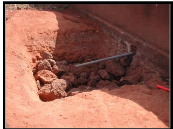
Figure 13. Earth and coarse gravel trickling filter implemented in Pampoyo
