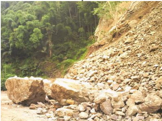
Figure 1. Rockfall cases occurred in the West Sumatra road ways. (Source: private documentation, 2011)
