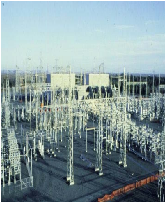
Fig 4. Nicolet convert station in transmission line Québec - New England
