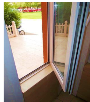
Figure.8.the window frame usage in Longson dormitory (Photo by author in 20th of April, 2014)
