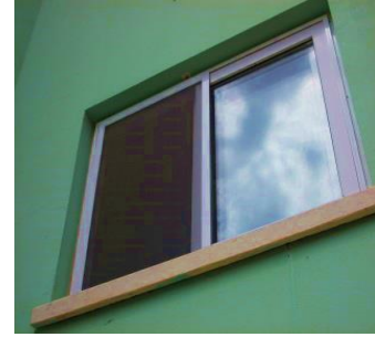
Figure 13. The window frame usage in Longson dormitory (Photo by author in 20th of April, 2014)
