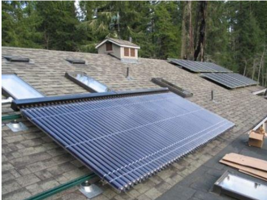
Figure 4. Solar water heater
