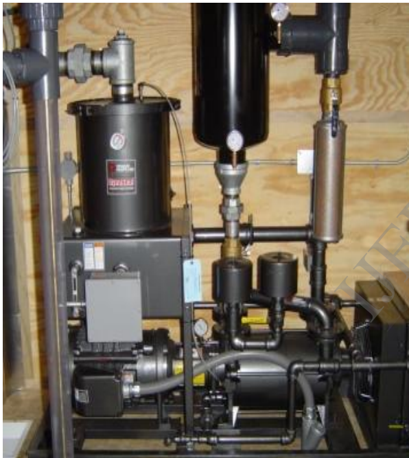
FIGURE 3 SET UP FOR DUAL PHASE EXTRACTION AT TRAVAINI LRP
