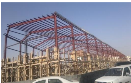
Picture (1) Taking into account the surrounding environment during the construction of the product
