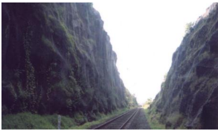
Fig. 3. Steep slopes in problem area
