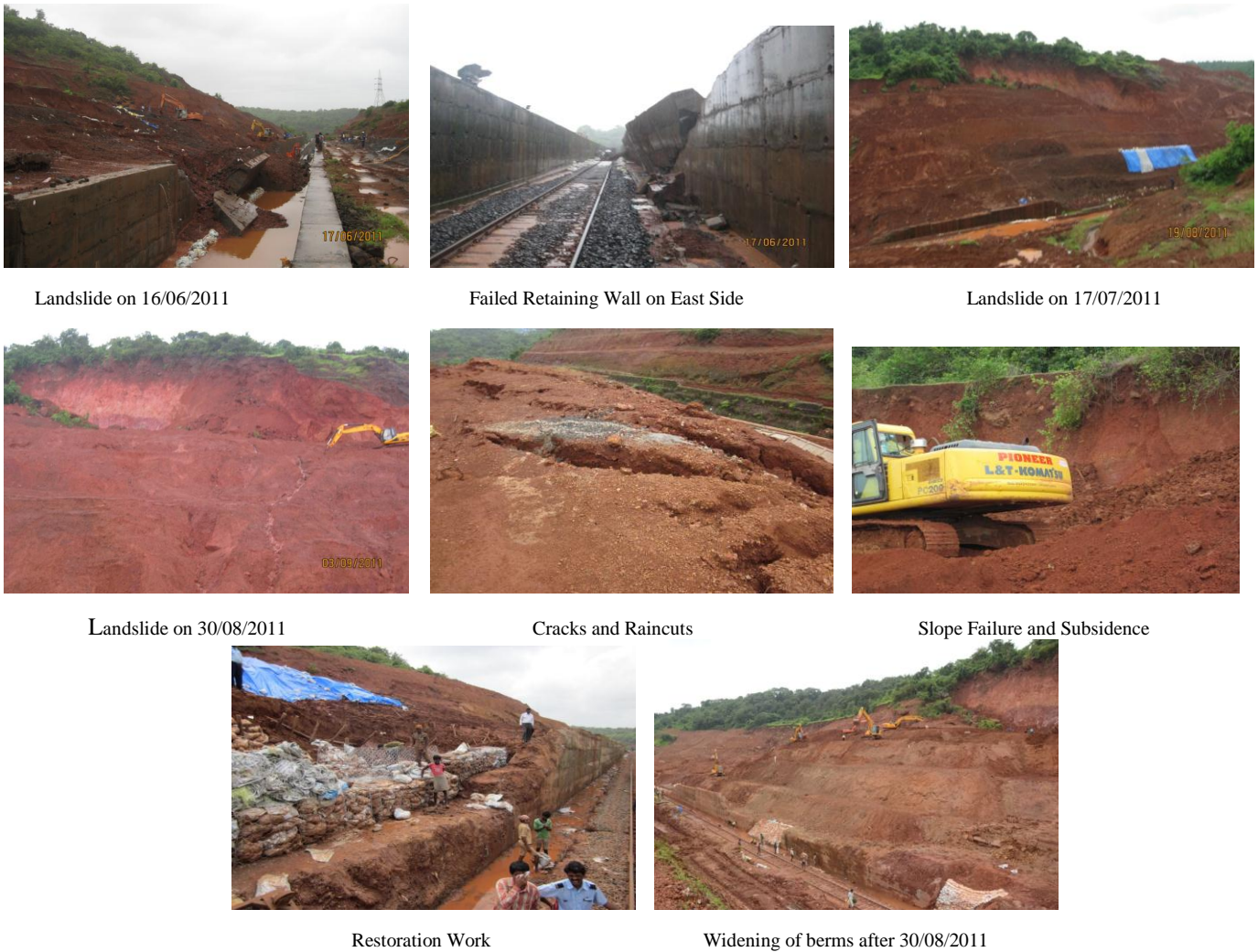
Fig. 6. Landslide during June – August 2011
