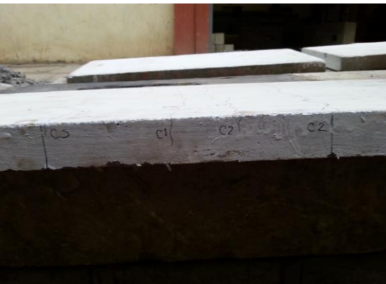
Fig 4: Crack pattern on the edge
