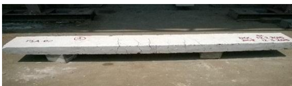
Fig. 22 Crack Pattern of GPC 0 % Ambient Cured Specimen.
