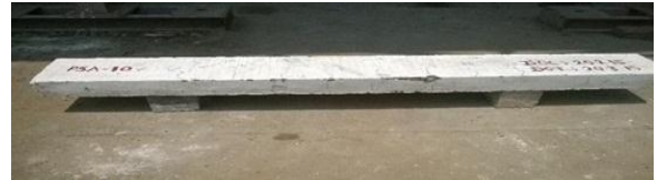
Fig. 23 Crack Pattern of GPC 10 % Ambient Cured Specimen.
