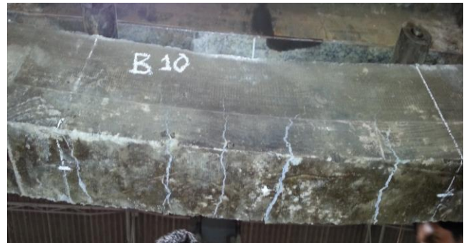
Fig. 12. Typical multiple flexural cracks at the bottom
