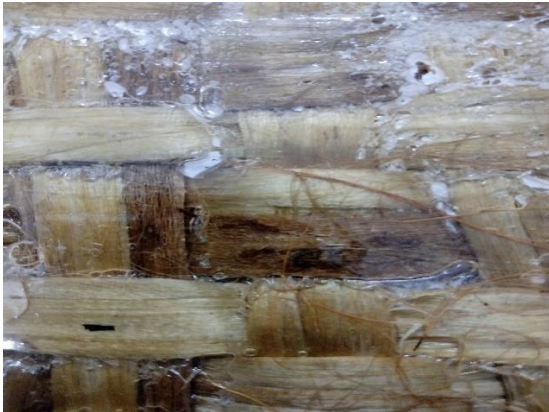
Figure 3.2 Improper Resin Application
