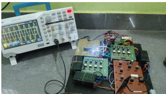
Fig. 21. Experimental test bench setup showing the low-voltage scaled prototype of the proposed 8-switch 31-level asymmetric multilevel inverter.
