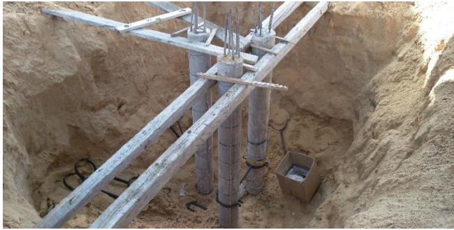
Fig. [18] Vertical Alignment of the Piles for Group (3) – Group of Three Piles
