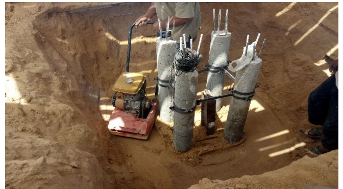
Fig. [22] Placing Compacted Soil around Tested Pile Groups for group (4) – Group of Four Piles
