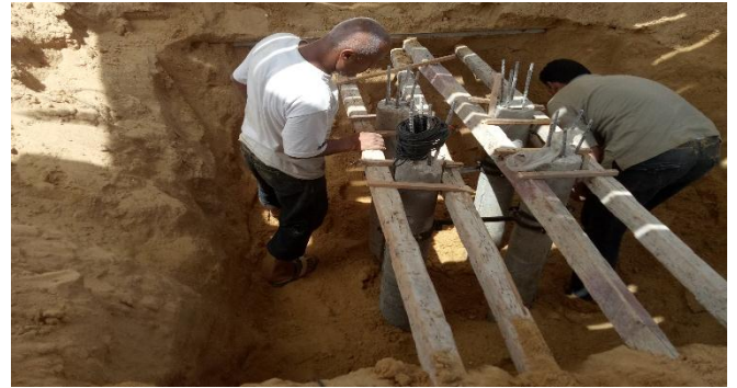
Fig. [21] Vertical Alignment of the Piles for Group (4) – Group of Four Piles
