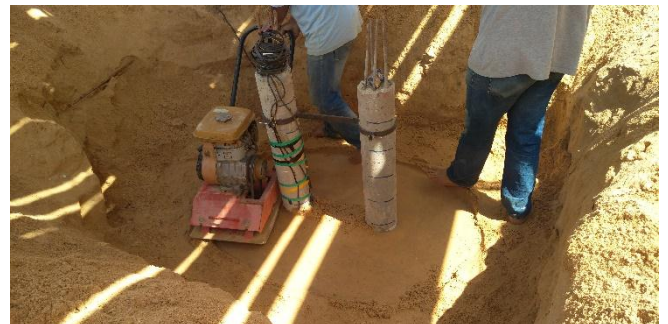
Fig. [16] Placing Compacted Soil around Tested Pile Groups for group (2) – Group of Two Piles
