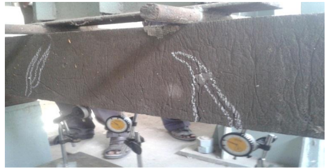
Fig -4: Failure mode of RCC beam
