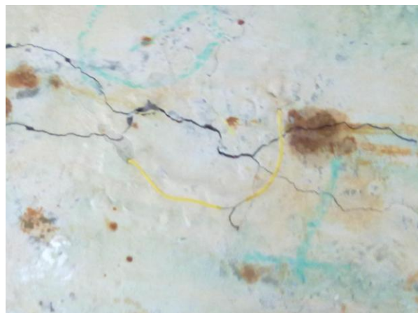
Figure 8. Crack Pattern on Specimen
