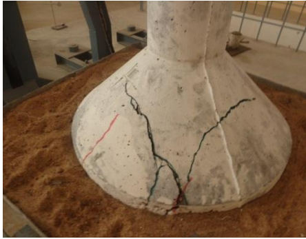
Fig 9: Crack pattern in Conical shell footing
