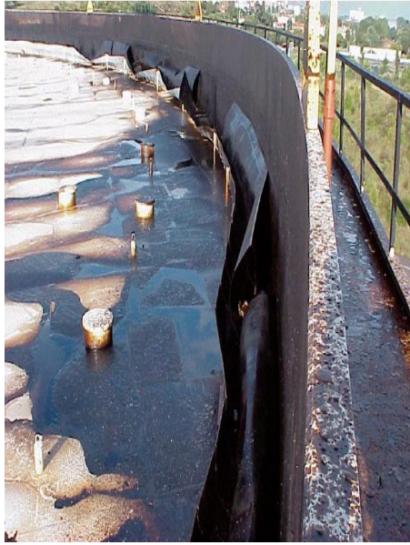
Fig. 2. Damage seals of a tank from the sloshing of stored Liquid.
