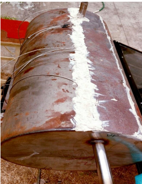
Fig.4 Thermal energy storage (TES) tank
