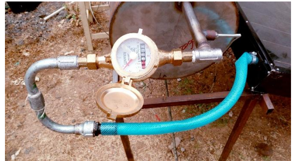
Fig.7 Flow meter to measure the rate of flow of HTF.
