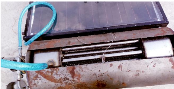
Fig.5 Inner view of TES tank
