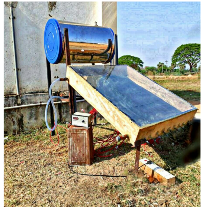
Fig (1) Parallel variable diameter riser tubes solar water heater
