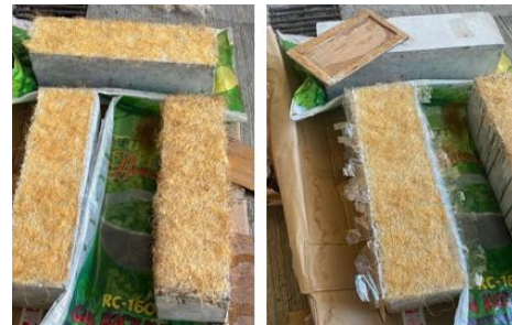
Fig. 6: Application of two-layer epoxy-externally bonded coconut husk fiber reinforcement on the beam soffit
