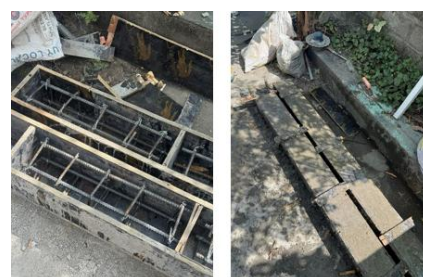
Fig. 7: Longitudinal and stirrup reinforcement arrangement of the beam specimen prior to external fiber application
