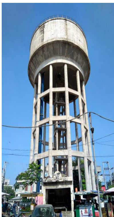
a) Water tank -1.
