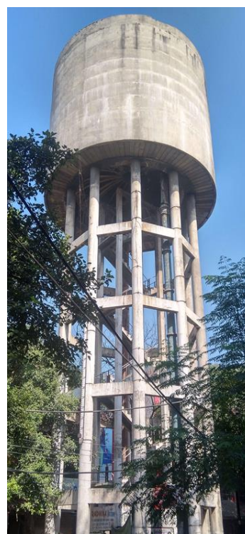
c) Water tank -6
