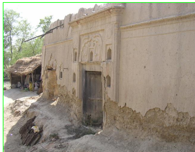
Figure 2: Capillary Rise in Water-logged Area, growing unhygienic living conditions (Sultanpur District)
