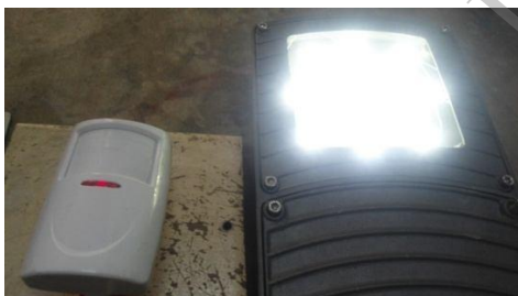
Figure 7. Primary and Secondary Circuit's LED – switched on
