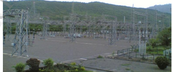
Fig. 1 Switch yard of Barn Grid Station
