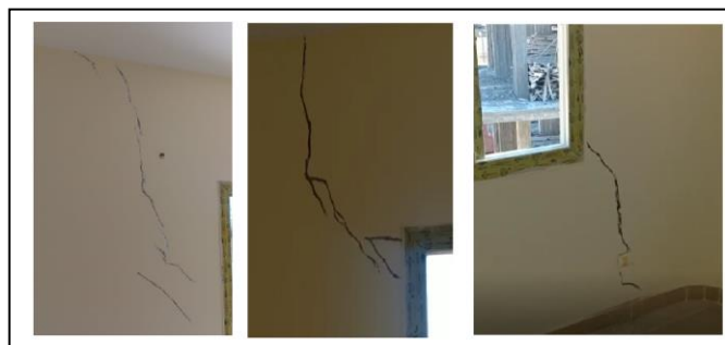
Figure 1 Architectural, other walls, Fence and structural problems in study site.
