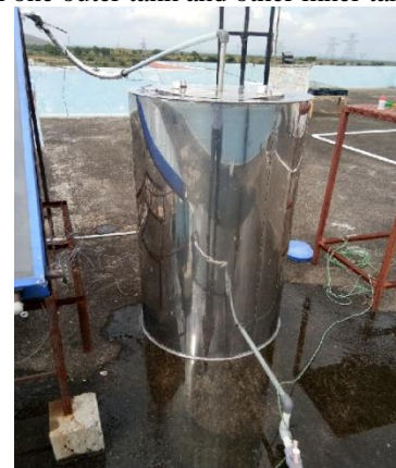
Fig.2 Thermal storage tank
