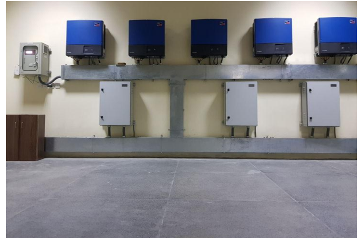
Figure 9 Inverters, distribution panel and cluster controller
