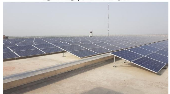
Figure 6 Solar panel field showing different blocks
