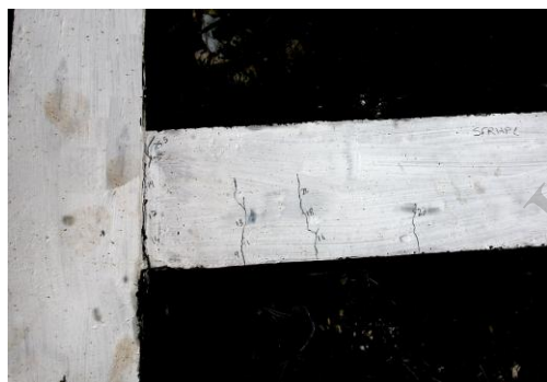
Figure 4. Failure pattern of SFRHPC beam column joint subjected to cyclic loading
