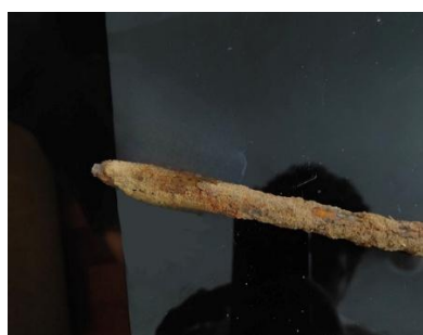
Fig.2 (a): Heavily corroded 10 mm \phi bar
