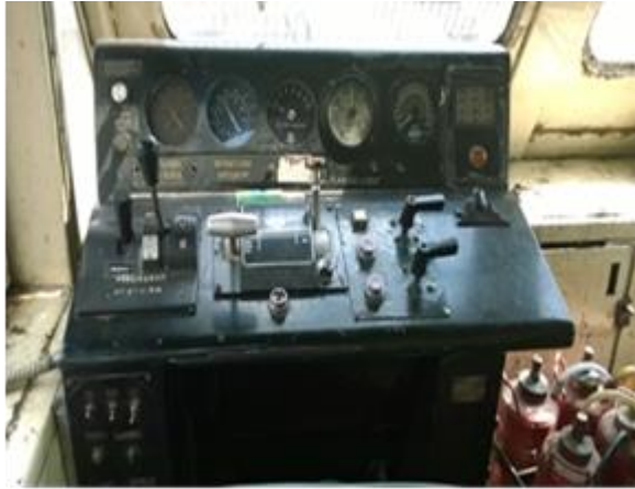
Fig. 7 Existing control panel of the WDP 4 model of the locomotive
