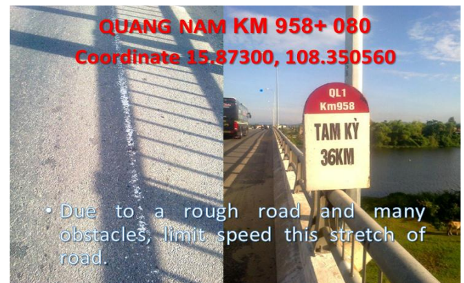
Figure 14. Warning result at KM 958+ 080 diocese of Quang Nam
