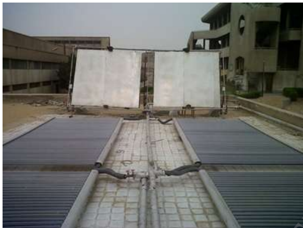
Fig. 5. Evacuated tube collectors under exposure of heliostat
