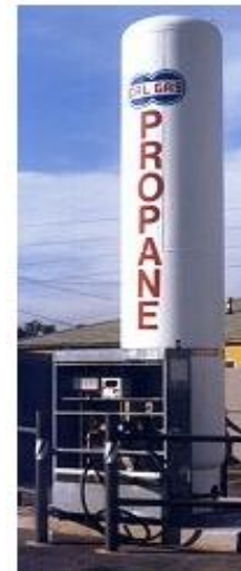
Figure 1: Vertical propane tanks
