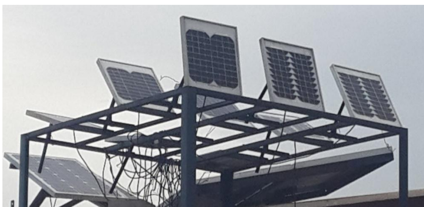
Fig. 2 Arrangement of the solar panels at different elevations
