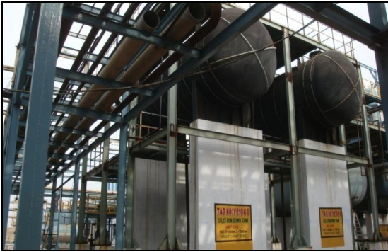
Fig 5 Methyl chloride rundown tank
