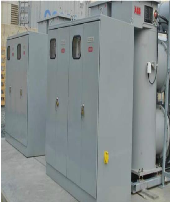
Fig.1 Control Panel for every bay in GIS
