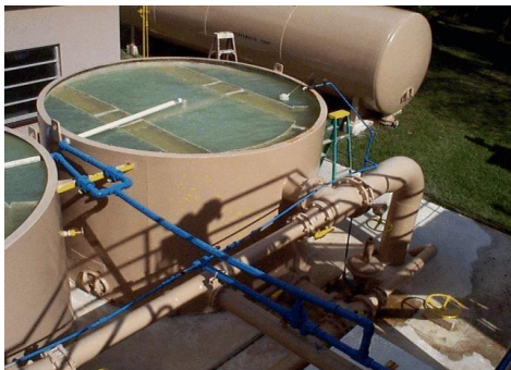
Fig.5. Rapid sand filter
