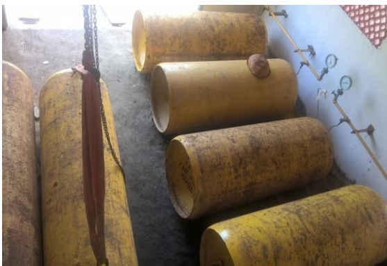
Fig.6. Chlorine containers stored in chlorine room
