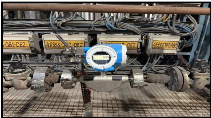
Figure-1 : New Promass Coriolis Flow meter installation.
