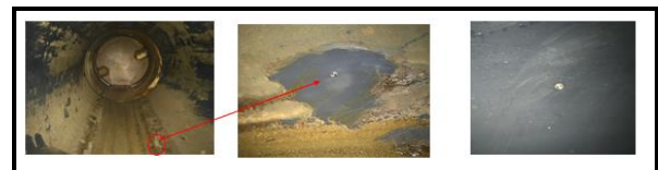
Figure (2) Gel mixer unit showing dirty pipe
