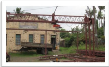
Fig. 3.2 Complete assembly of crane
