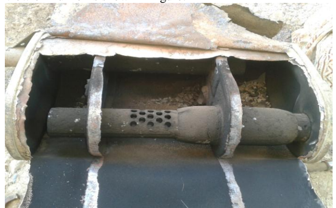
Figure 3- 2 Inside view of existing muffler
