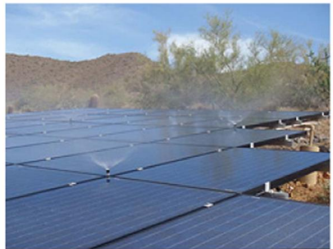
Figure 25. Setup of water sprinkler cooling system [21]
