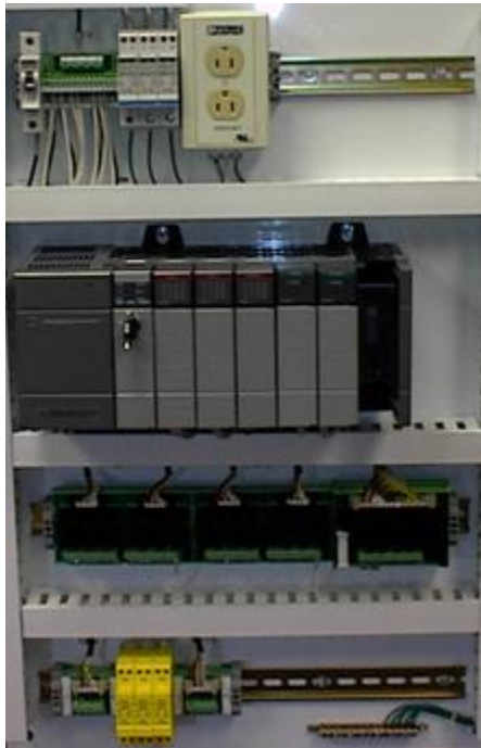
Fig. 5 A rack type PLC
