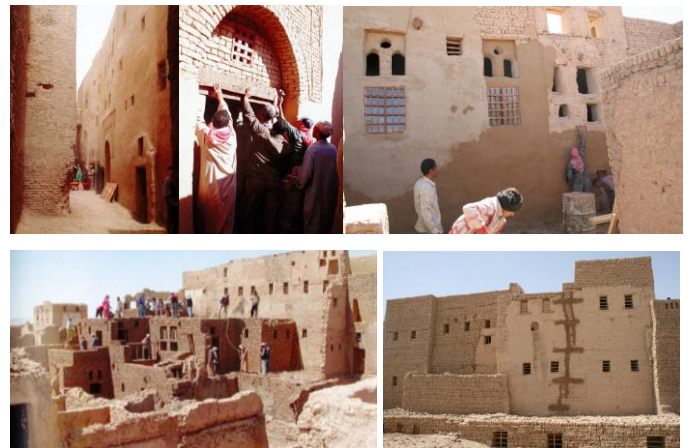
Fig. 6. Conservation, restoration and reconstruction of the Shihabiyya quarter in Qasr Alakhla Oasis [6] [7]
