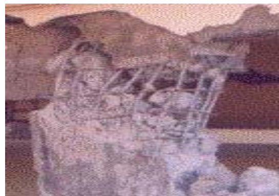
Figure 1 (a) failure at construction Joint.
