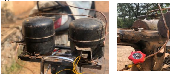
Fig:D. Compressors and Control valve
