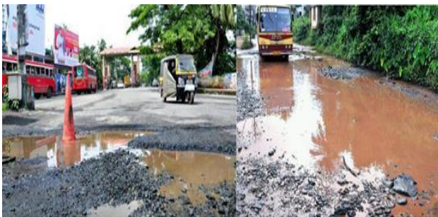
Fig 2 Deteriorated bituminous pavement [2]
