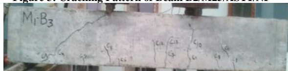
Figure 4: Cracking Pattern of Beam B3/M25/AST2/NF
