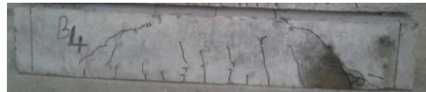
Figure 5: Cracking Pattern of Beam B4/M25/AST2/NF
