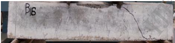
Figure 17: Cracking Pattern of Beam B16/M50/AST2/WF/1.5%
