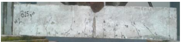
Figure 16: Cracking pattern of beam B15/M50/AST2/WF/1%
