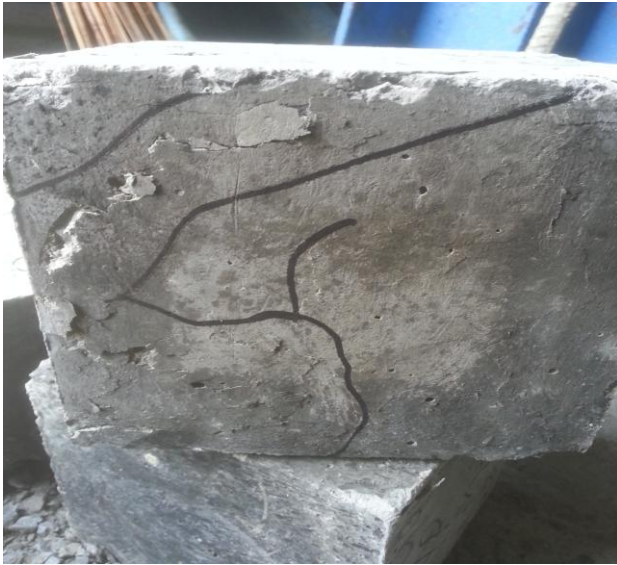
Fig. 9 Visible cracks on cube after testing
